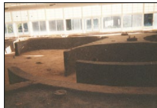
Construction of indoor pool at Bogan Park in 1997, the first pool in the county to be enclosed in a permanent structure.
